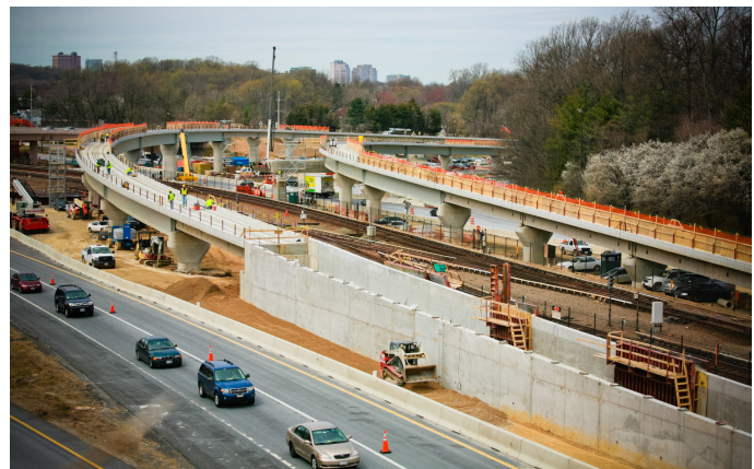
Figure 1 - New Silver Line Connection to the Existing Orange Line in the Median of I-66.
